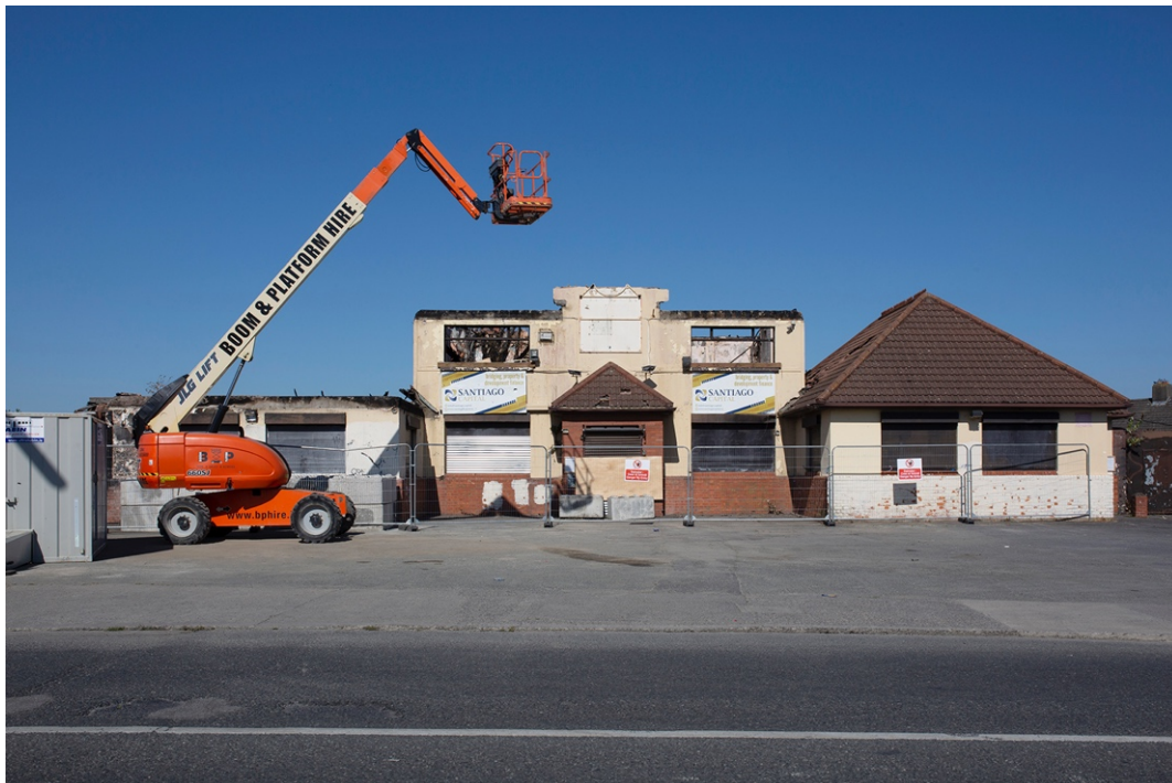
Figure 4.19: Matts of Cabra pub shortly after fire, Fassaugh Avenue, Cabra. Source: Mandy O'Neill, 2022.
