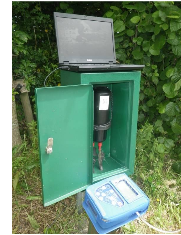
Above: GEN3 system during deployment setup to Kinsale road landfill perimeter well, Cork, Ireland.
